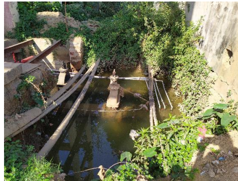
Leakages at the OHT
